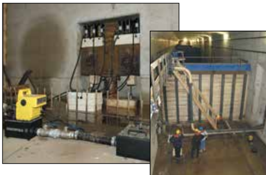
◀ Enerpac lightweight aluminum RAC-506 cylinders are ideal for wet environments such as this tunnel under the river (Holland High-Speed Train Line).
